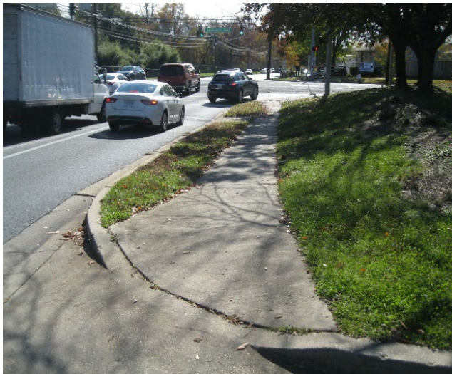
Figure 1 - Non-ADA compliant sidewalk ramp
