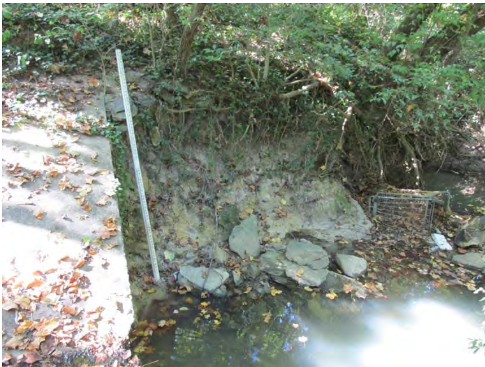
60-2. 09/28/2017: Outfall 60, facing south. Looking at erosion around the end of the concrete channel.
