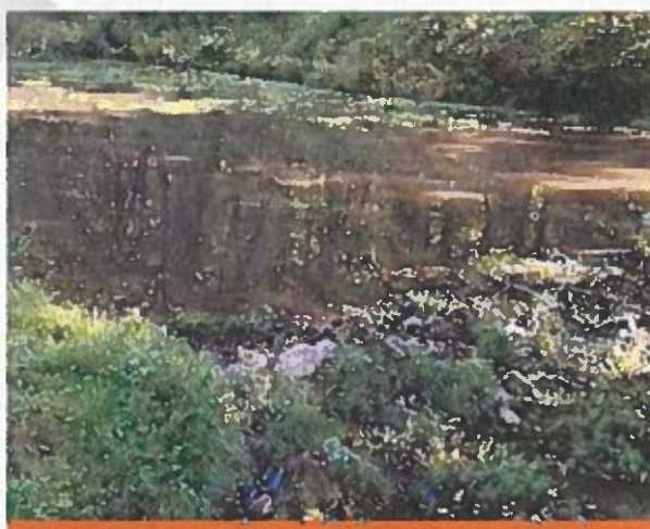
FIGURE 10 Greenbelt Lake forebay.
