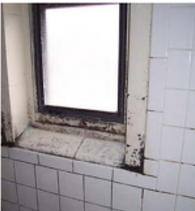
Livability: Mold due to moisture at bathroom window.
