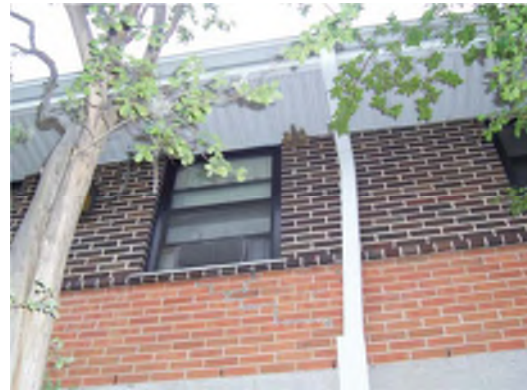
Tubes above for bat evacuation through building.
