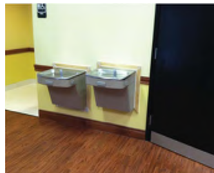
Accessibility: Community room hi/low drinking fountain exceeds 4" max protrusion depth along accessible path.
