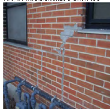
Structural: Stress cracks present; filled with concrete mix, but will continue to increase in size over time.
