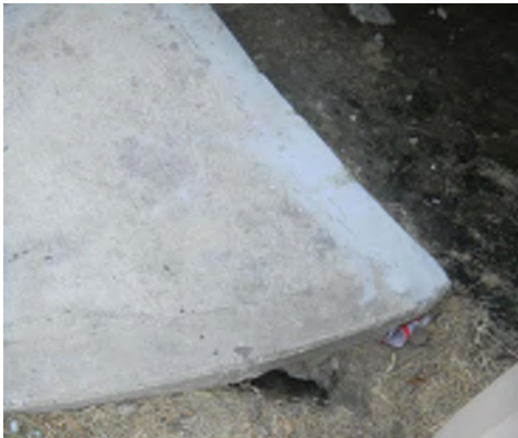
Water leak under sidewalk.
