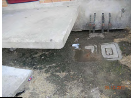
Water leak under foundation and sidewalk.
