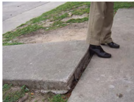
Life Safety/Accessibility: Heaved lead walk poses a tripping hazard @ Building 11.
