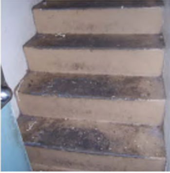
Life Safety: Interior concrete stairs do not have tread covers to prevent slipping.
