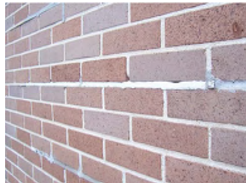
Structural: Stress cracks present; filled with caulk, which provides no structural value; will continue to increase in size overtime.
