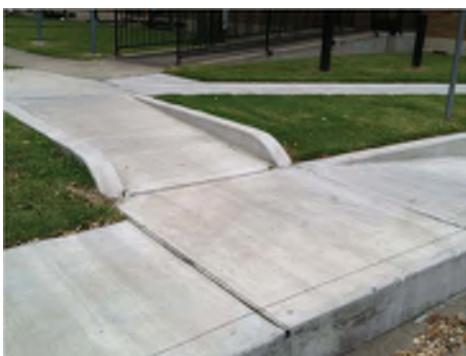
Life Safety/Accessibility: No curb along landing @ 6" drop-off; provide curb at drop-off to parking.
