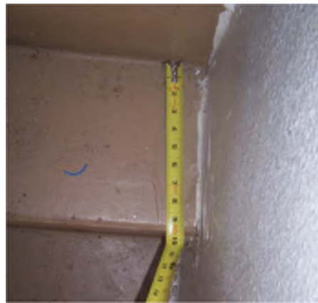
Life Safety: Interior concrete stairs do not meet minimum rise: run standards; does not meet minimum head height clearance.
