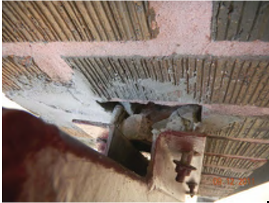
Steel rail separation – close up.
