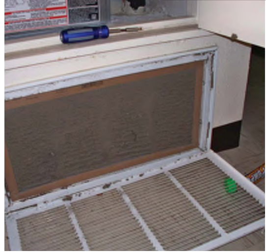
Return air filter/grill at floor
