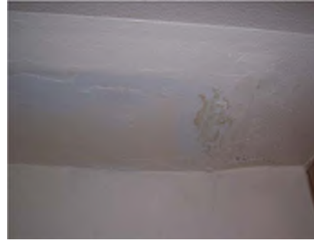
Health/Safety: Evidence of plumbing leaks in kitchen ceiling from 2nd floor bath fixtures above.
