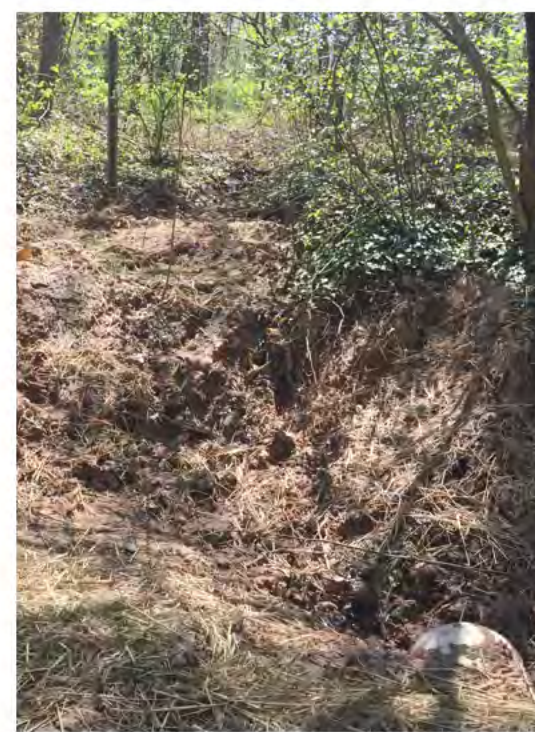
C - This photo, actually taken within Stand 4, is indicative of Northway's typical roadside condition within Stand 11. The roadside ditch isn't stabilized with vegetation, which otherwise would provide erosion control and runoff control.
