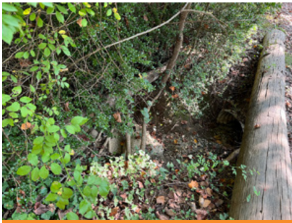
FIGURE 29 Sedimentation at outfall to the east side of lake
