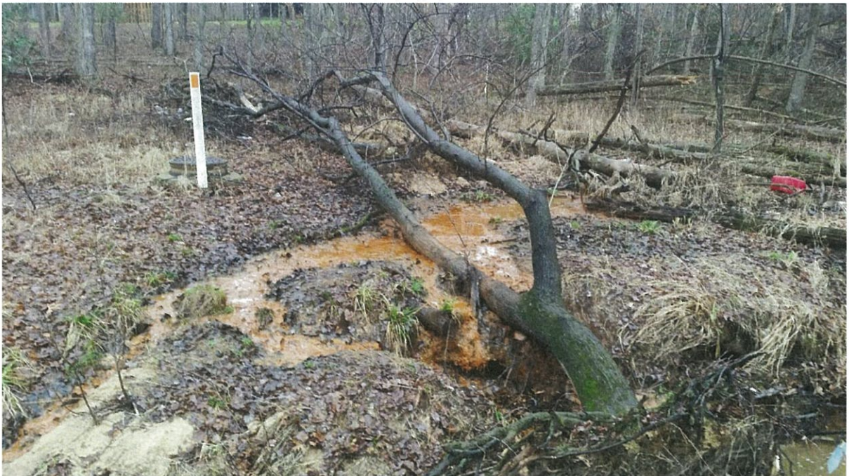
View of possible sewer leak along Reach 3. Notice the discolored runoff near the sewage manhole.
