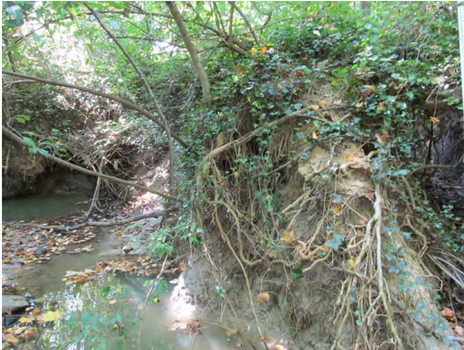
60-6. 09/28/2017: Outfall 60, facing north. Looking at eroded channel downstream.
