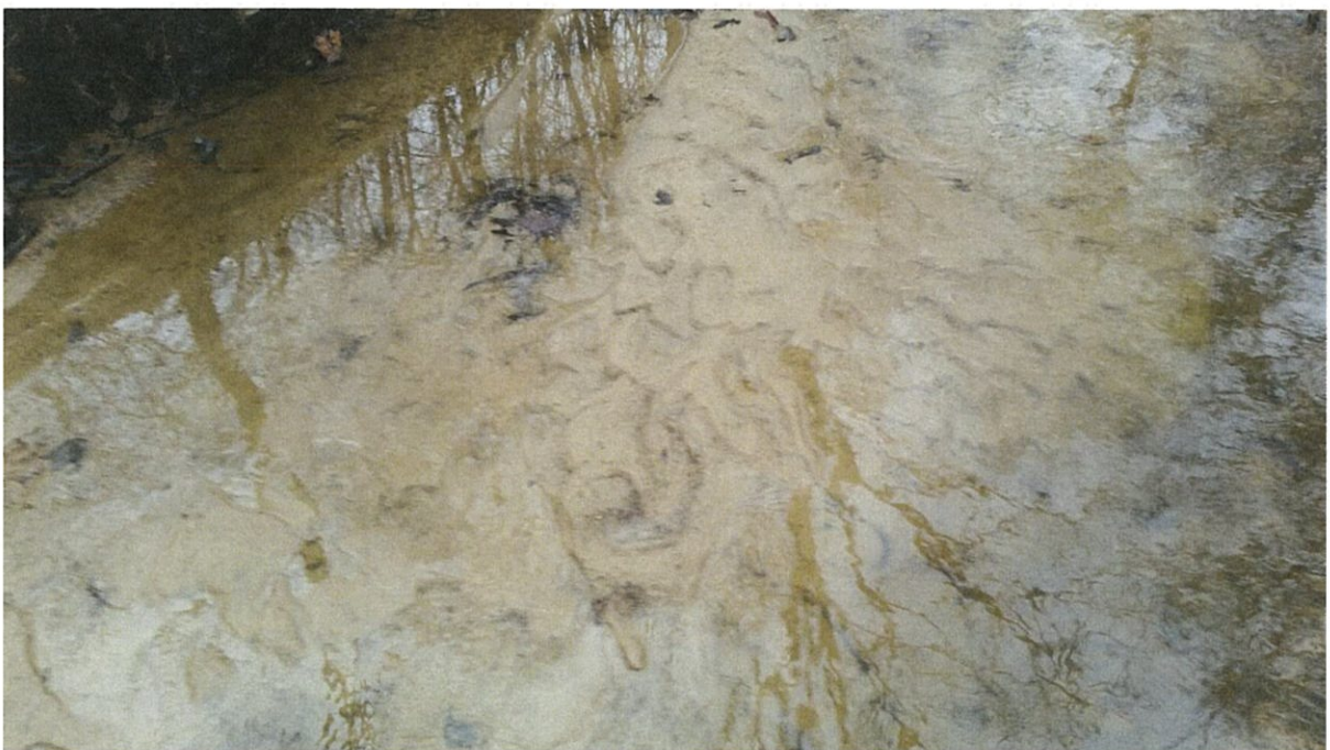
View of sand bottom along Reach 2. The streambanks in this reach are actively eroding.
