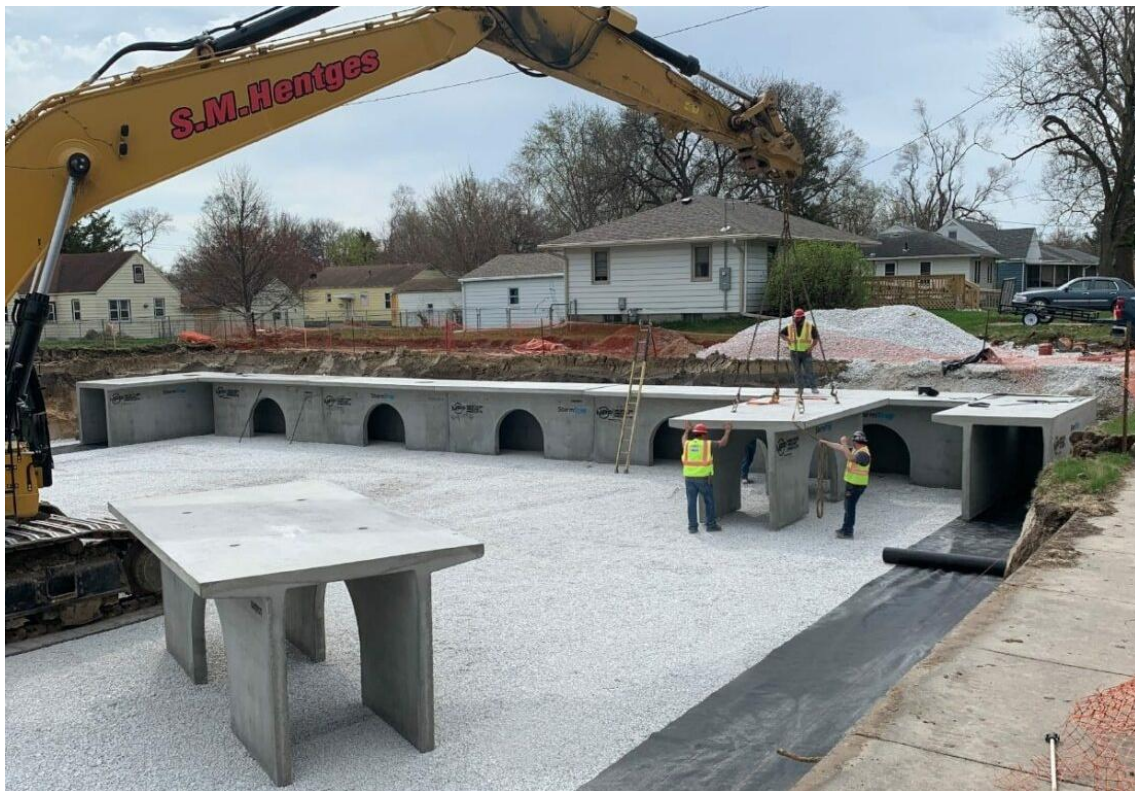
Figure 20: Example of an underground detention system being built in Des Moines, IA. Image courtesy of StormTrap website (stormtrap.com).
